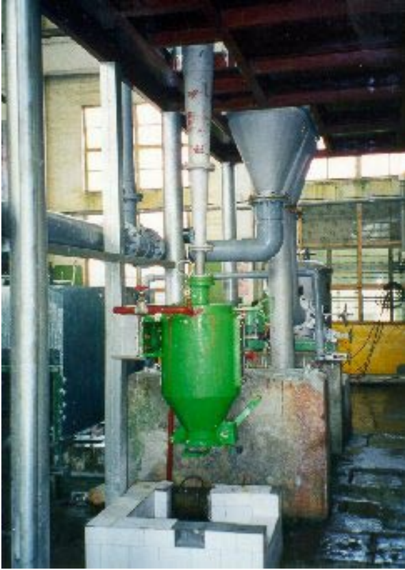
Photo 22: Sand removal system
