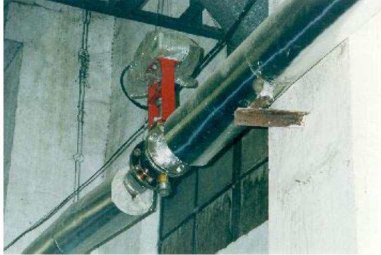
Photo 23: Steam pressure control valve
