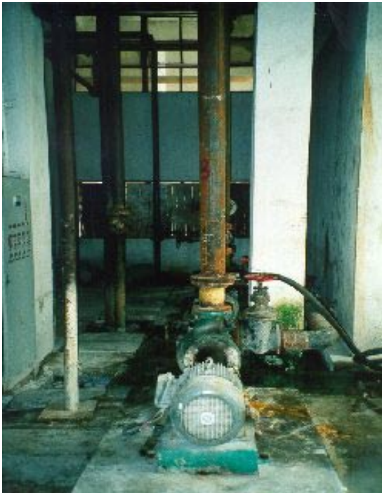
Photo 16: White water recycling pump
