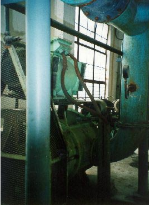
Photo 14: 90 kW motor used for cardboard machine vacuum pumps
