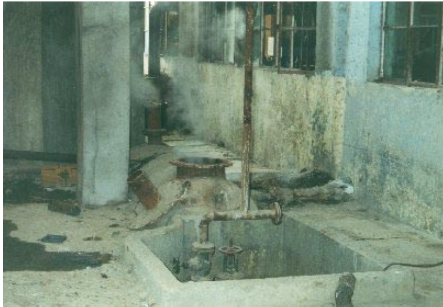
Photo 12: Condensate recovery piping system
