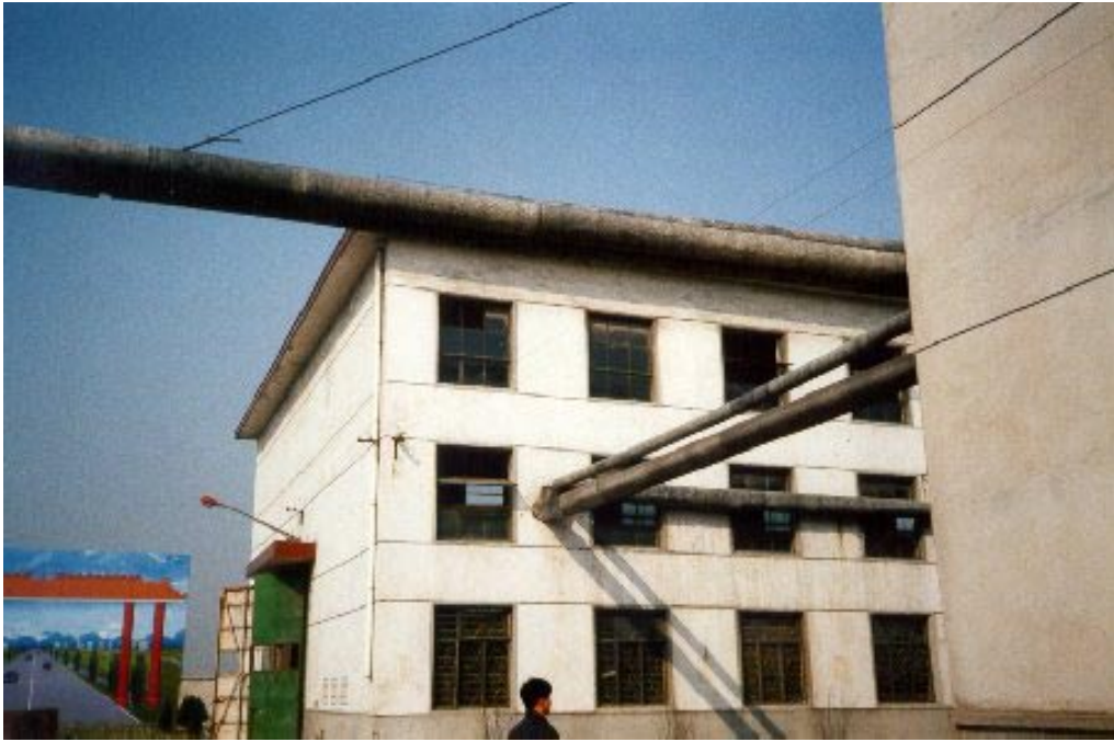
Photo 9: Steam pipes insulation
