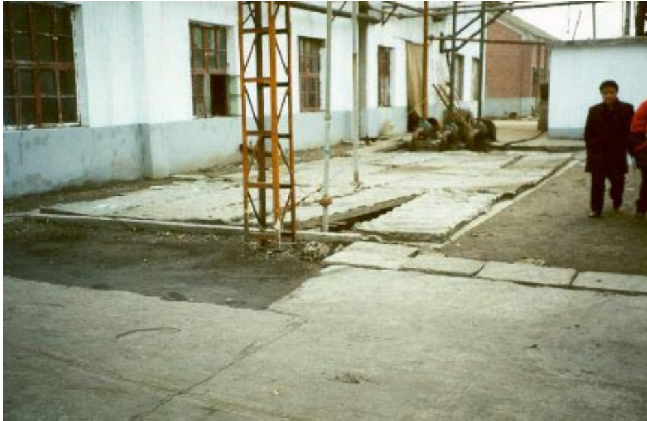
Photo 5: White water clarifier basin
